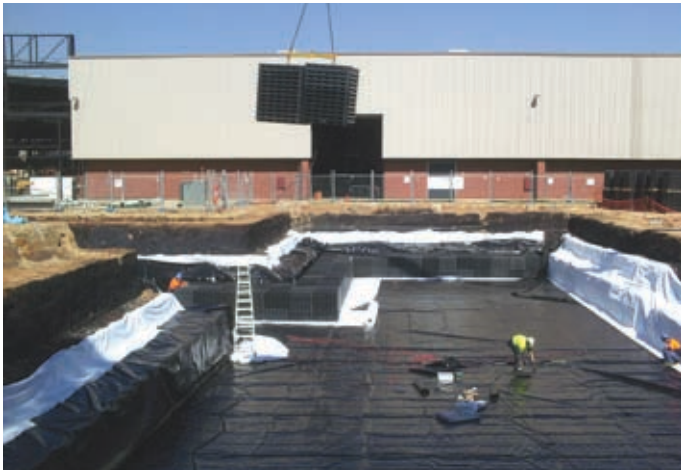
Day 2 5.00pm Weld three piece liner and begin outer wall construction. Rainstore 3 cells craned in.
